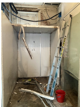
Above: Years of water damage & an old fireplace revealed.
