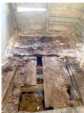
Above: Water logged, rotted flooring.
